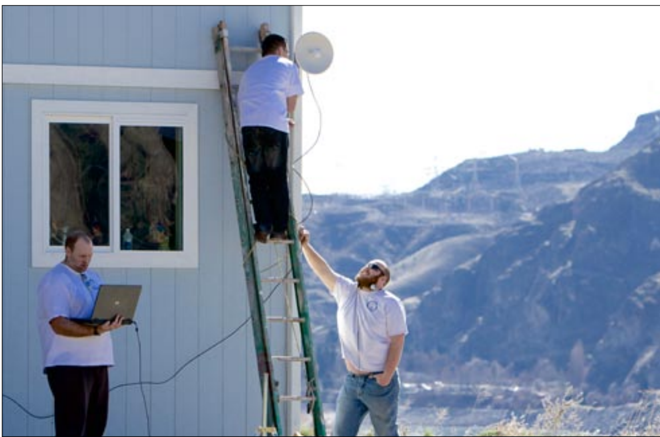
From left, Brad Oliver, Victor Camarena and Micah Seekins install a new connection and relay at the home of Cory Christman on a hillside north of Elmer City. Christman said it was taking him 10 minutes to download a Youtube video. Download speeds were nearly 1,200 percent faster after the install. — Scott Hunter photo
