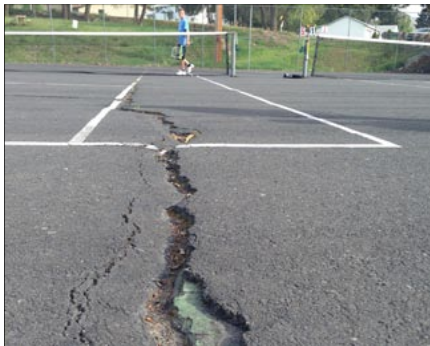
Cracks in the tennis courts rendered two courts useless this year. will begin this week and take about two weeks to finish before demolition can begin. Carlson said the projects will
