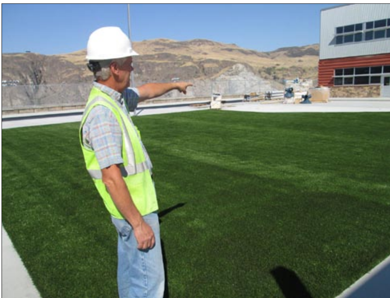
Roger Easing, who supervises the K-12 school construction for the district, views an astro turf play area behind the new facility. It is one of several student areas for relaxation or play scattered throughout the project. The astro turf was laid down last week. — Roger S. Lucas photo
